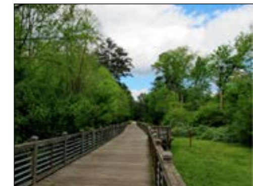
This 988-ft wooden boardwalk will be replaced with a pre-cast concrete called PermaTrak. Photo by Steve Bach.
