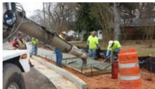
New sidewalks on Main Street created a more walkable environment for residents.
